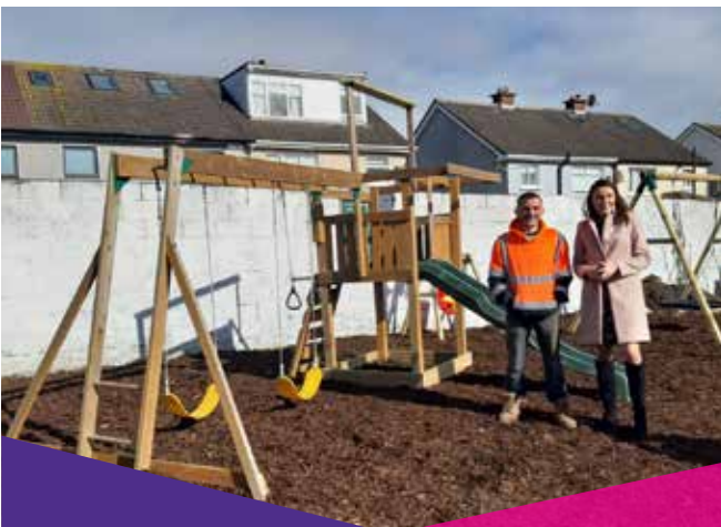
Collen Construction and Amazon embarking on a complete refurbishment of our garden, refuge centre
